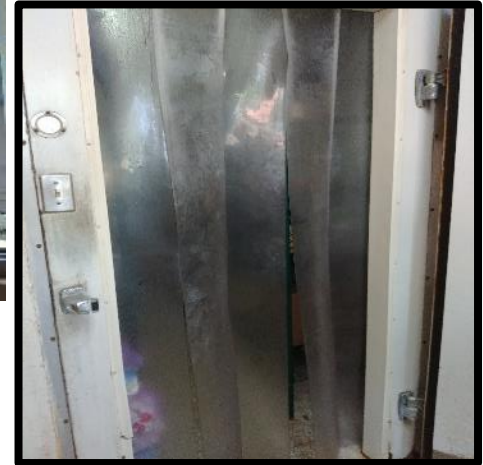
PVC strip curtains to reduce loss of air conditioned air
