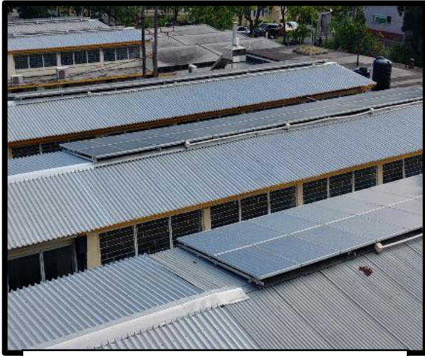
Solar panels on the roof of engineering building
