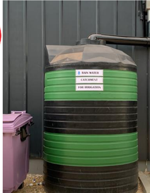
Rainwater catchment for Irrigation - Juici Head office
